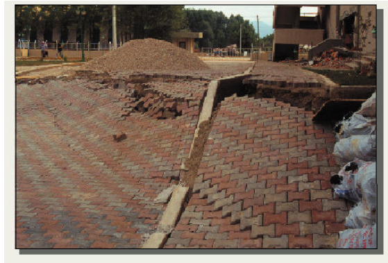
Figure 5. The effects of liquefaction in Kocaeli earthquake, 1999 (© http://www.koeri.boun.edu.tr/deprenmuhspeceals/kocaeli/kocaeli_eq.htm )
